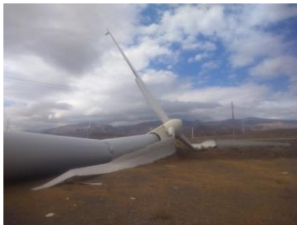
Fig. 1. Crash of the wind turbine tower in Manjil because of loosening of bolts
