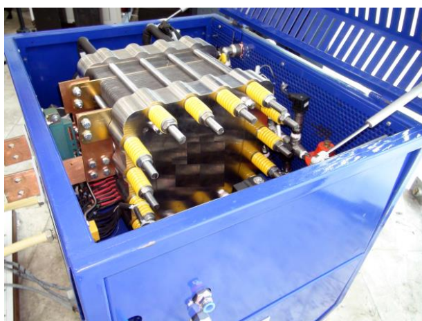
Fig. 2. Integrated power system for dead-end tests
